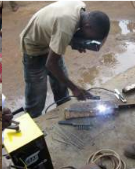
Figure 6 TREESPA welding machine being tested on site in Kilosa (ESAB THJ 140 arc welding machine)
